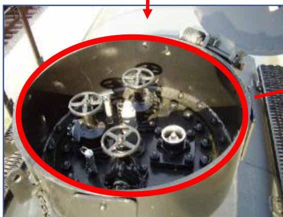
Valving inside the \frac{3}{4} " protective housing
